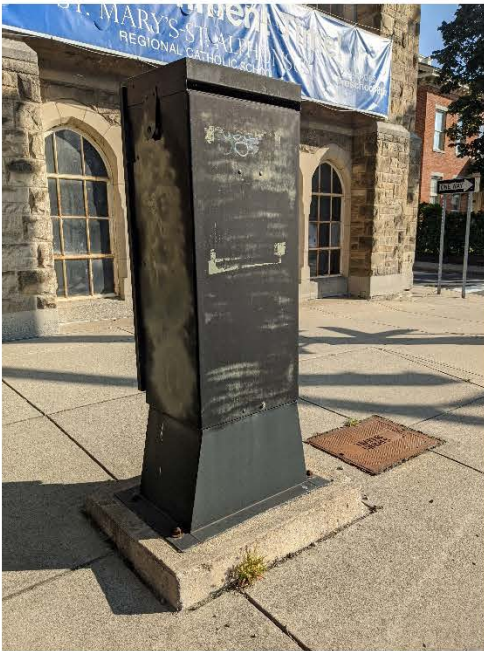
Corner of Warren and Church Street electrical box.
