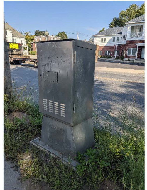
Corner of Warren and Oak Street electrical box.
