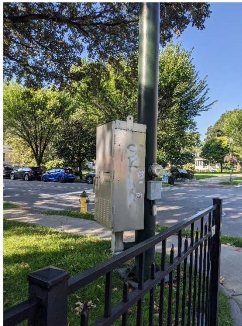
Corner of Ridge and Maple Street electrical box.
